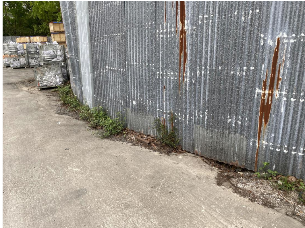
Photo 1: Hoarding without concrete footing
